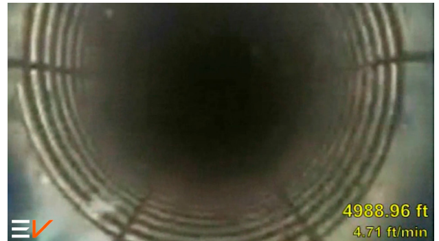
Figure 2: Downview footage of shortened camera assembly running through an overshoot
