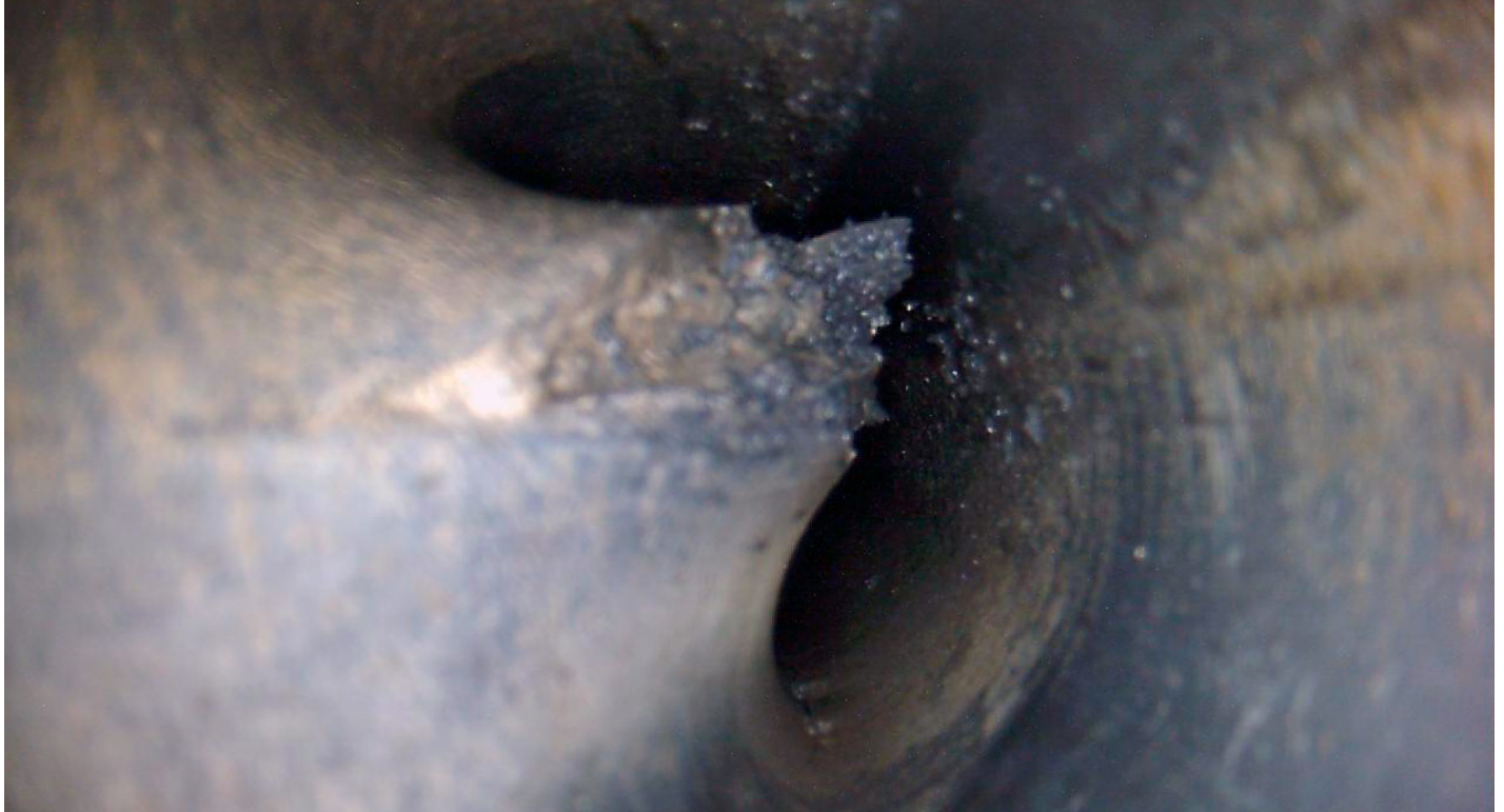
Figure 1: Extent of restriction preventing equipment access
