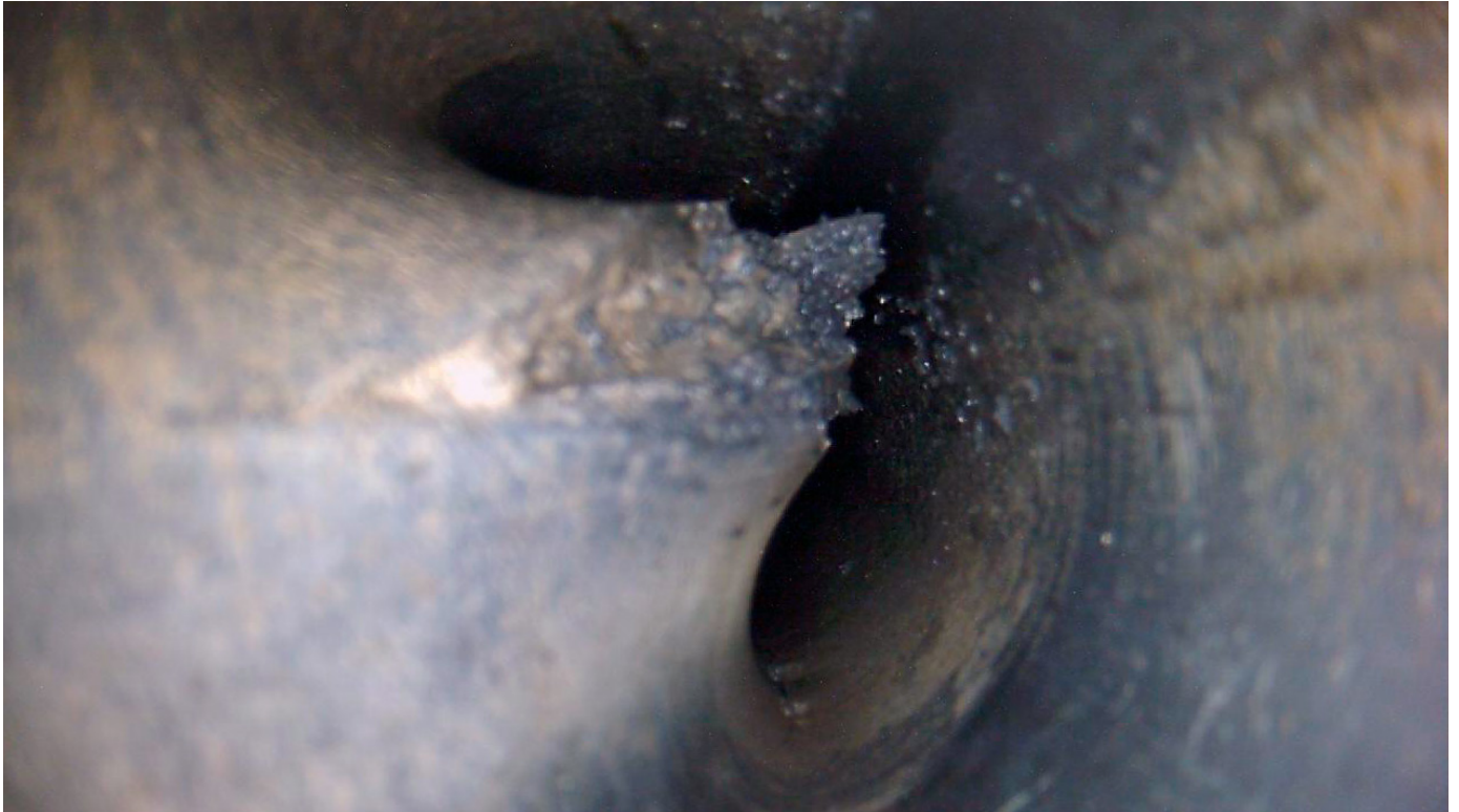
Figure 1: Extent of restriction preventing equipment access
