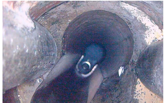
Figure 2: Impact damage identified from tool impact at SPM
